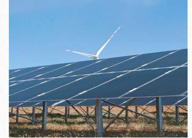
MALATYA ARAPGİR SOLAR POWER PLANT
